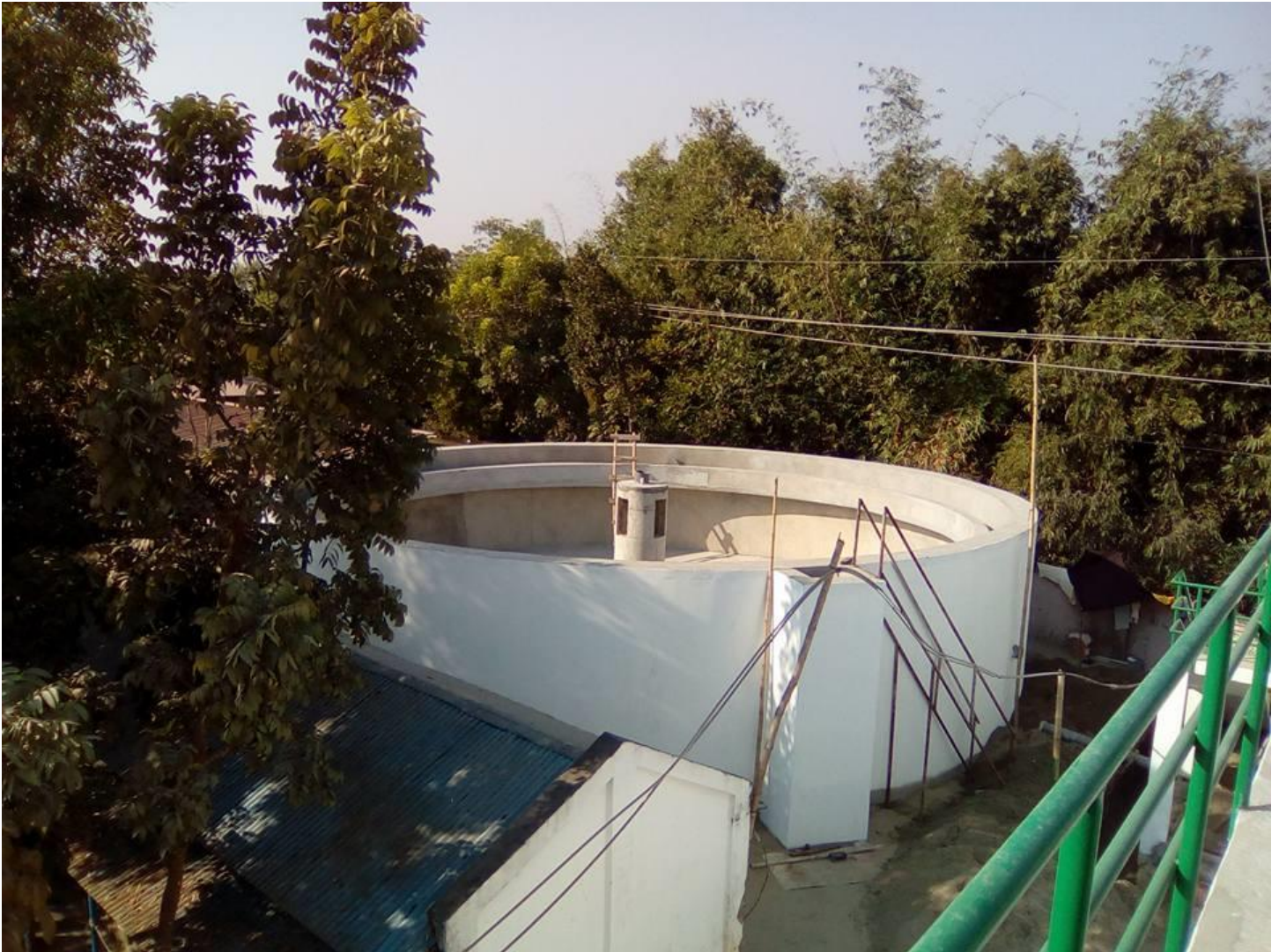
PICTURE-1 OF CIVIL CONSTRUCTION WORKS OF “ETP” COMPLETED FOR SAIHAM KNIT COMPOSITE LTD, NOYAPARA, HOBIGONJ
