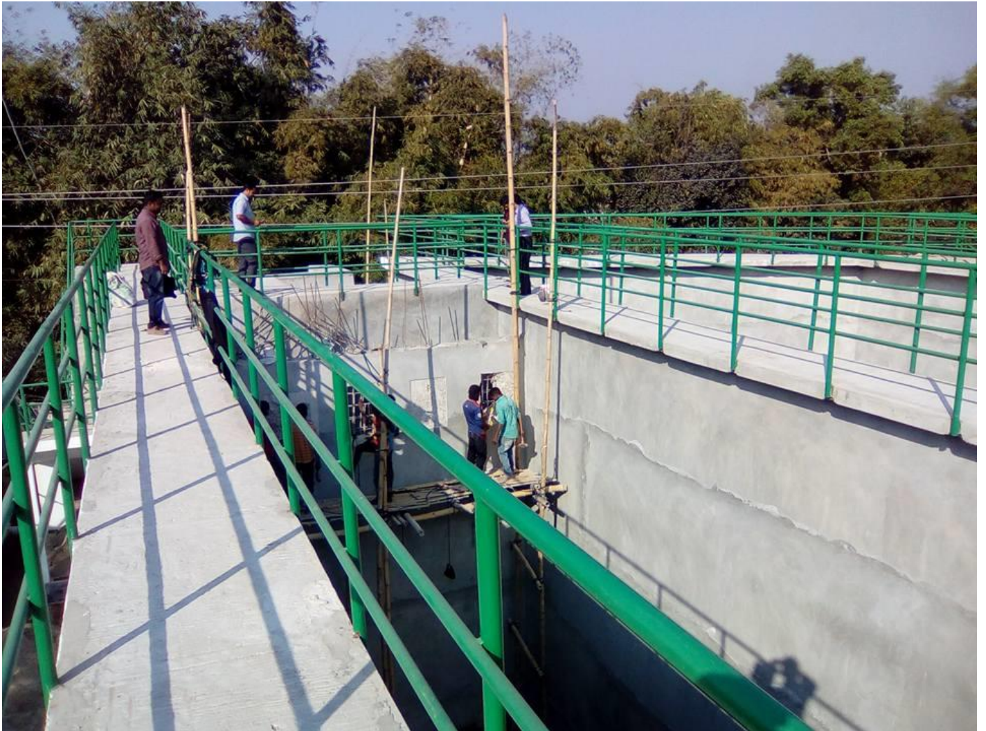
PICTURE-3 OF CIVIL CONSTRUCTION WORKS OF “ETP” COMPLETED FOR SAIHAM KNIT COMPOSITE LTD, NOYAPARA, HOBIGONJ
